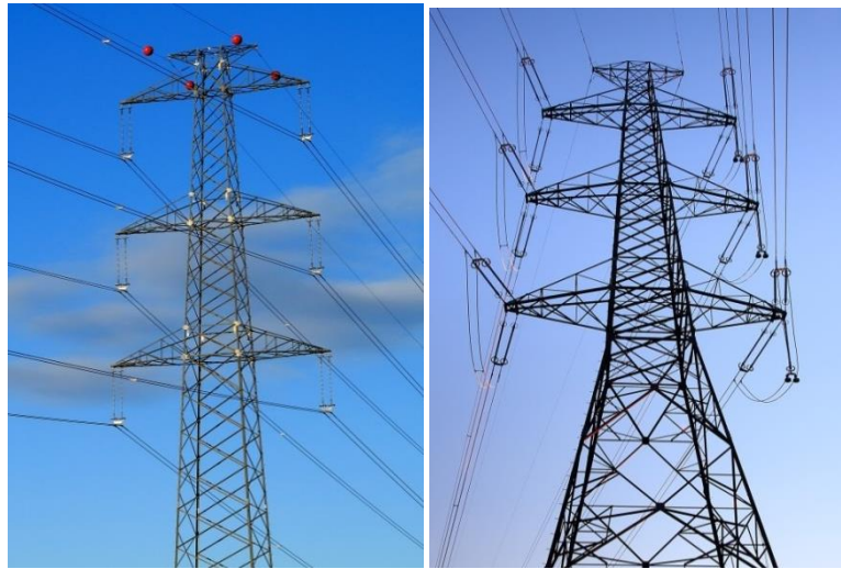
Figure 5-3: Line carrier pylons and anchor masts for 400 kV aerial conductor
