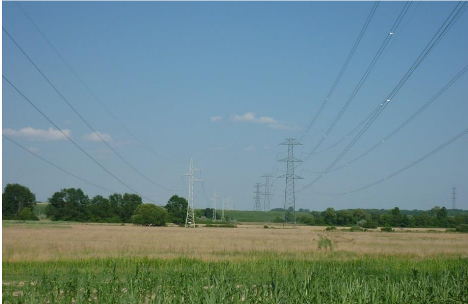
Figure 5-2: High voltage power transmission line designed in a wire corridor, implemented section
