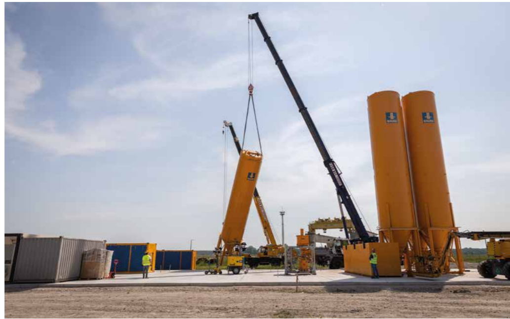
Two slurry mixing plants, constructed in the immediate vicinity of the site, provided the necessary cementitious and bentonite slurry for the cut-off wall and soil improvement works.
